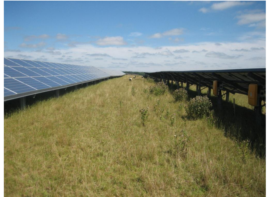
Photo 6. Grassland with thistle on bare patches beneath the panels, Site three
