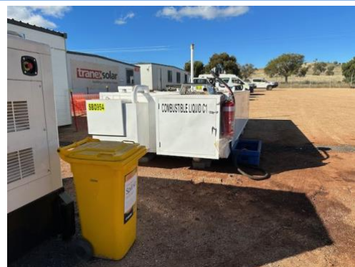
Photo 8: Bulk fuel tank, spill bund and spill kit.
