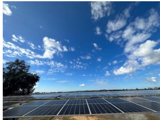
Photo 4: Installed solar panels.
