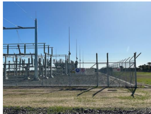
Photo 6: Substation with security and PPE signage.
