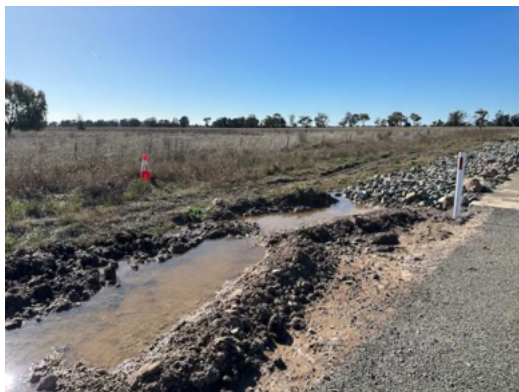
Photo 29: Incomplete works on Blands Lane.
