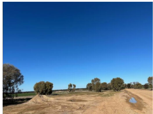
Photo 30: Incomplete works on Bodells Lane
