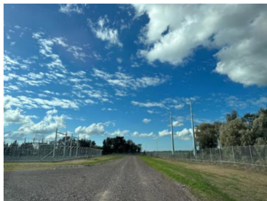
Photo 7: Substation, all-weather access track and perimeter fence on Myers Lane (Left to right).
