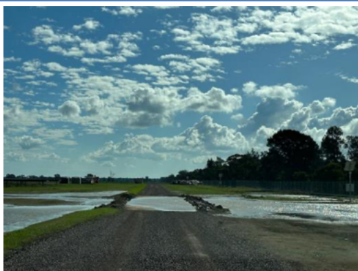
Photo 23: Low-lying access track crossing allowing water flow.
