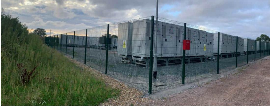
Insert 43: Example of Part of a BESS and Bund (example from Herfordshire)
