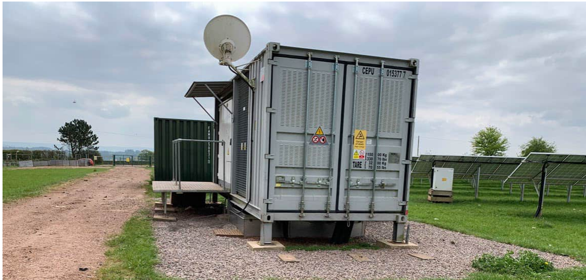
Photo 10.4: Example of a Typical Inverter
