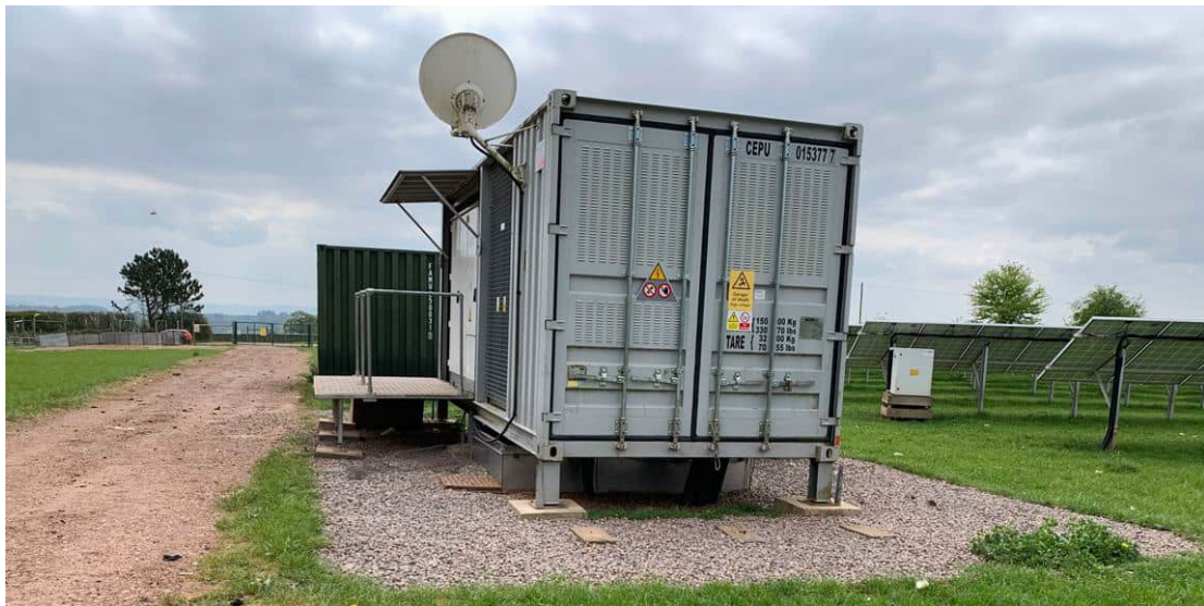
Inserts 19: Typical Inverter Container (example from Monmouthshire)
