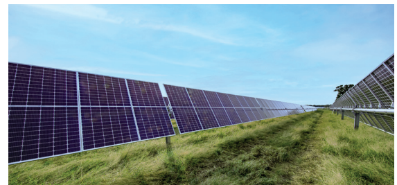
Solar panels are mounted on posts, enabling growth of vegetation underneath that allows for natural drainage and the interception of storm water
