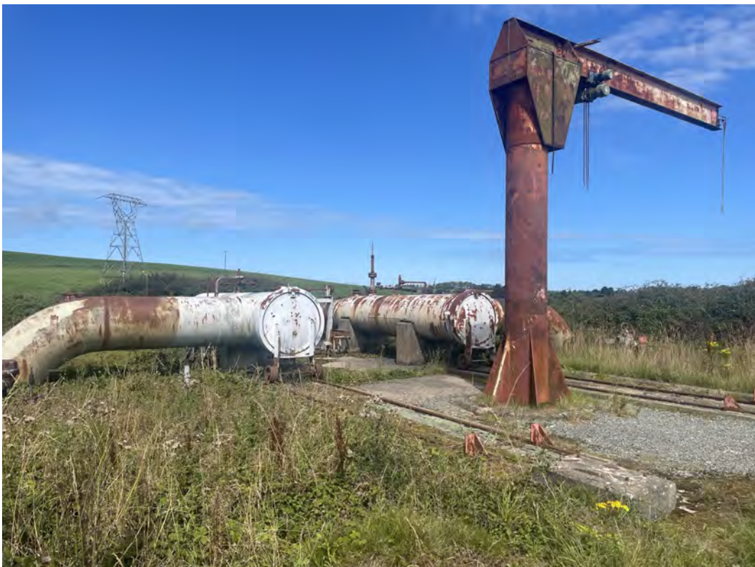
Photo 8—Remnant pipework remaining on site.
